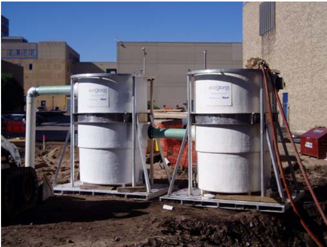
ecoStorm plus unit without filter (right side) used as an upstream holding tank. ecoStorm plus unit with filter (left side) used to treat dewatering prior to direct discharge into an existing storm sewer.
