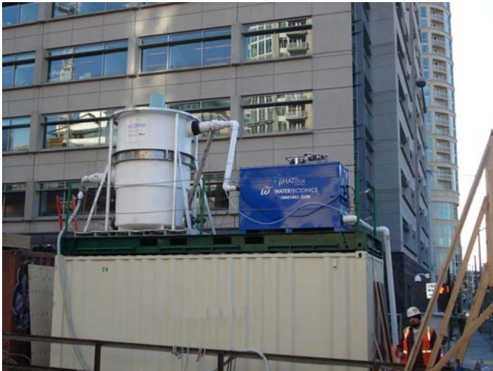
ecoStorm plus (upstream) working in conjunction with a PH adjustment technology (pHAT) box (downstream) in a major downtown construction dewatering site.
