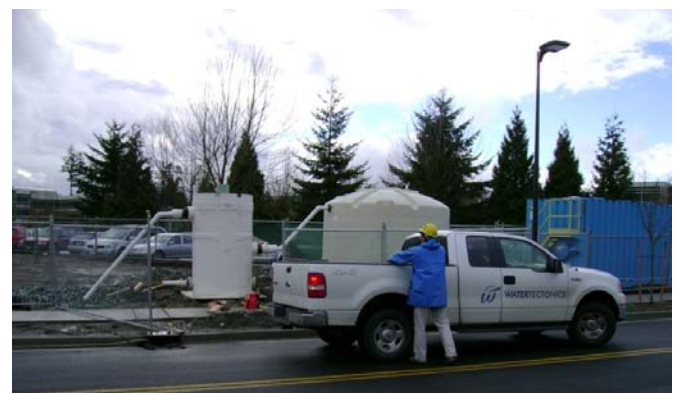
ecoStorm plus with upstream storage tank on new construction dewatering site with direct discharge to sanitary sewer.
