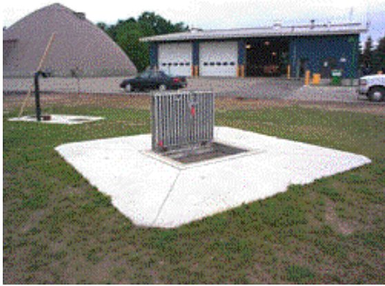
ecoSep installation at a NYSDOT maintenance facility
